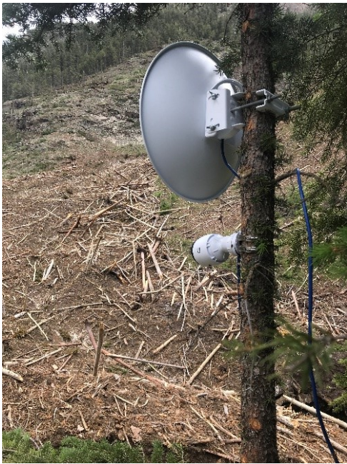
Figure 7—Equipment at Henson Creek
